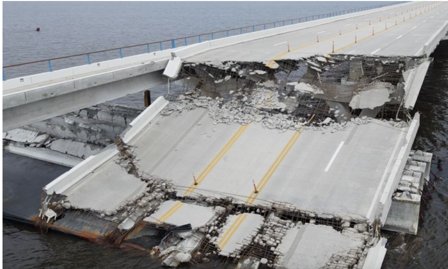
Figure 24: Three Mile Bridge over Pensacola Bay collapsed during Hurricane Sally 84
