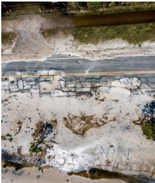
Figure 33: Impact of Hurricane Michael Storm Surge on US 98
