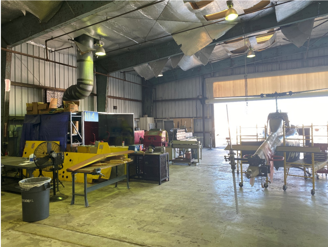
Picture 2 Hangar ceiling in disrepair
