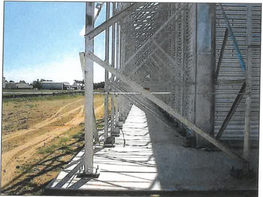
The GRE frame features extensive cross bracing to provide sufficient wind resistance relative to the height of the structure.
