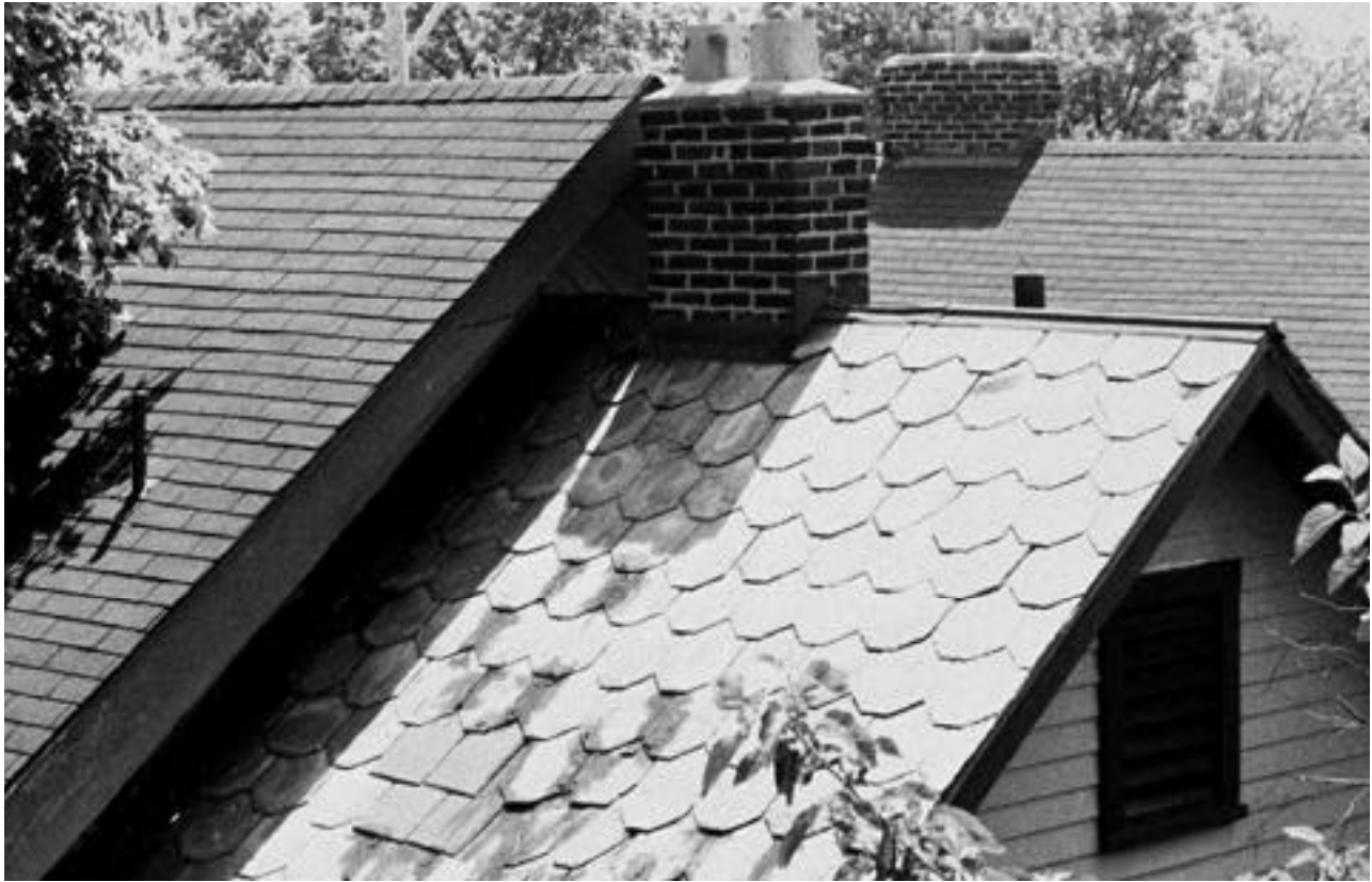
This slate roof should be carefully investigated since it has a makeshift repair. Other problems include the chimney, which is too low, and the vent pipe, which is too narrow.
