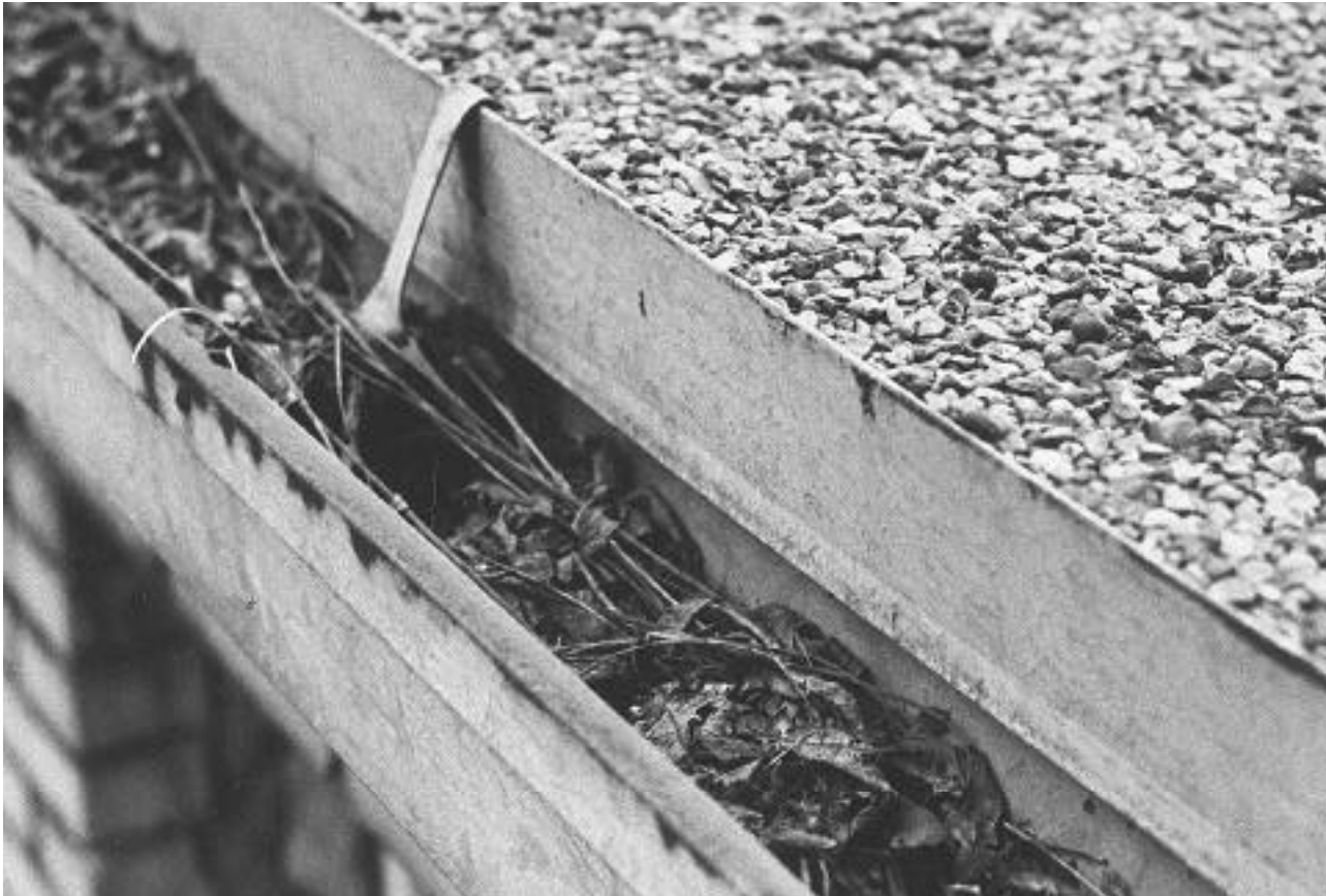
The gutters on this low-slope roof are deteriorating largely because of the accumulated detritus that they hold. They should be inspected and cleaned periodically.
