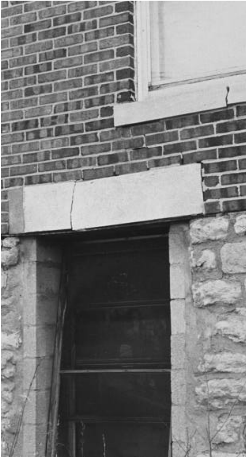
Failure of a concrete lintel and sill due to differential settlement of the building. Permanent repairs will be quite expensive. Note the makeshift shoring of the lintel.
