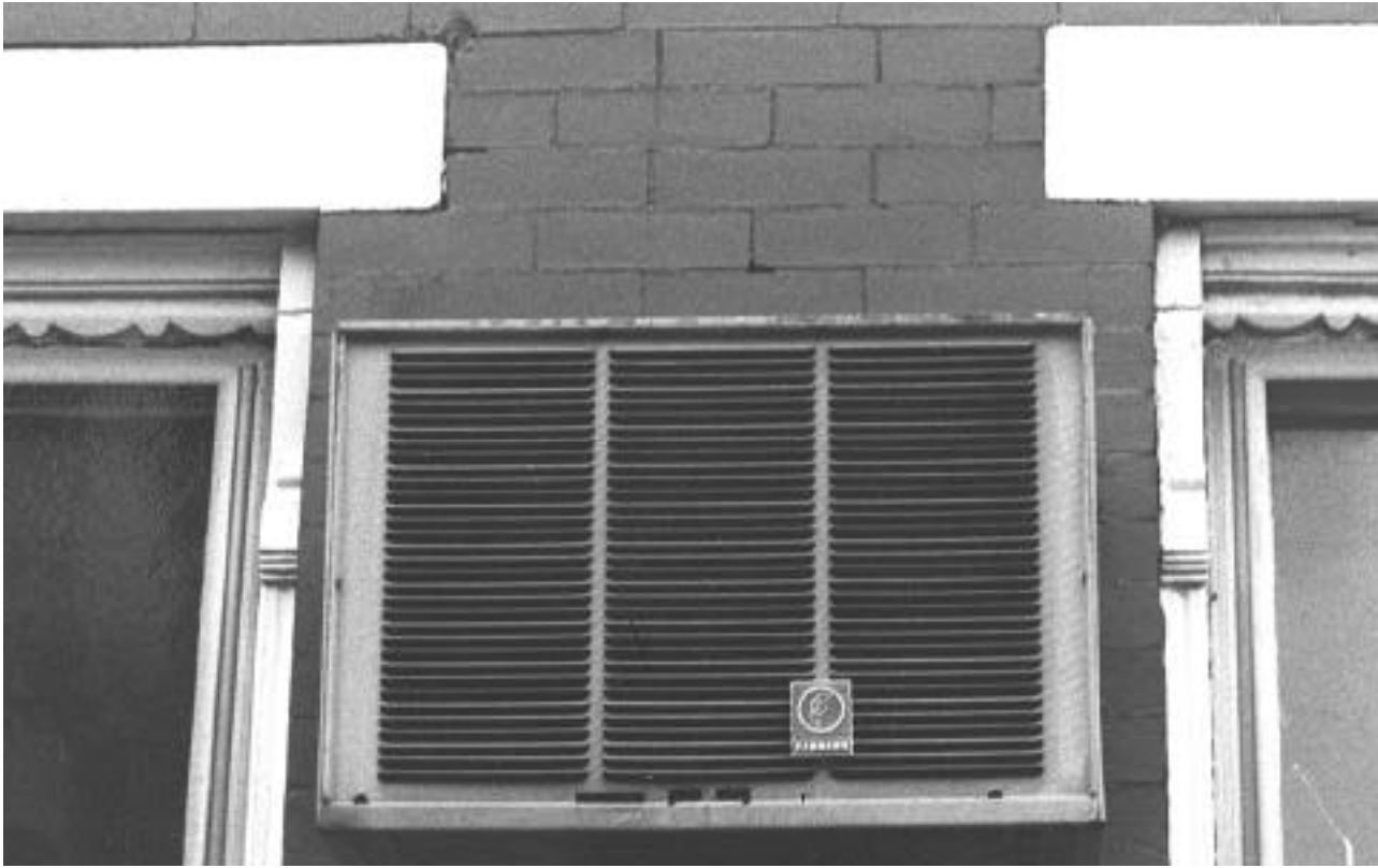
Installation of this air conditioner destroyed the structural integrity of the bearing wall between the two windows.
