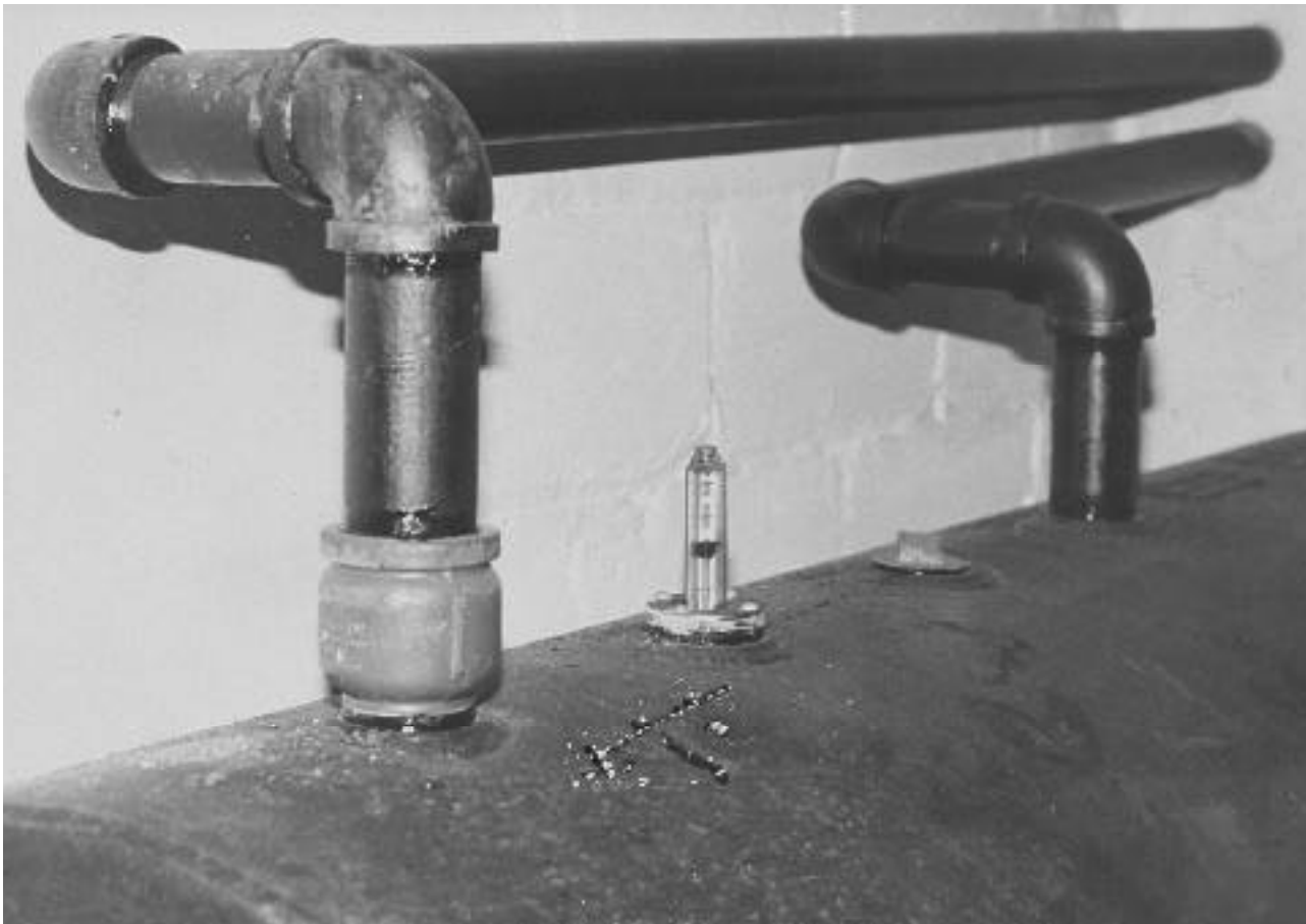
Look for signs of corrosion around and within oil storage tanks and check the operation of the oil level gauge. Use a dipstick to check for signs of condensation in the tank.
