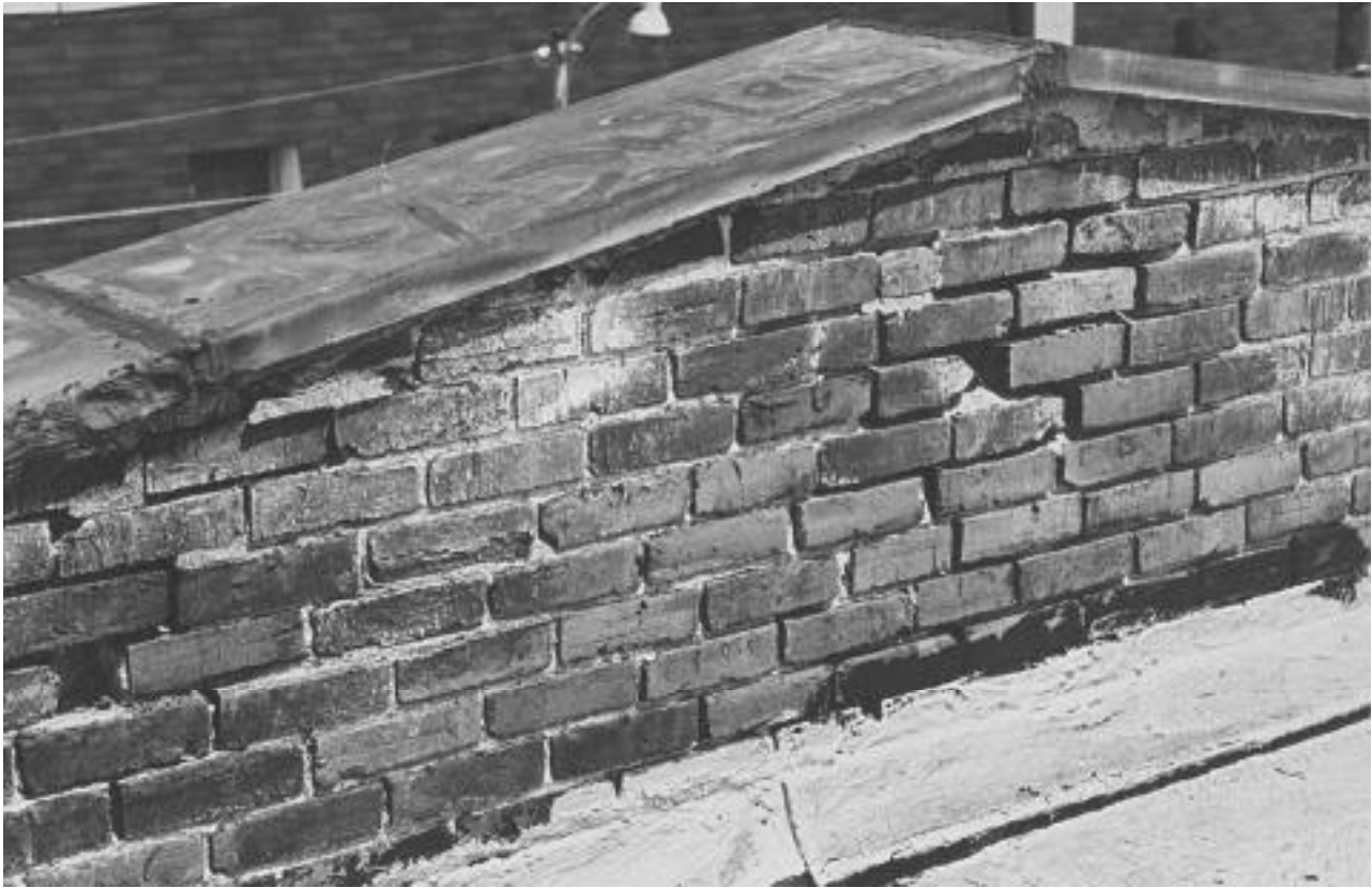
A deteriorated parapet wall that badly needs repointing. Fortunately, the wall has not yet exhibited serious movement, but it will if left unrepaired.
