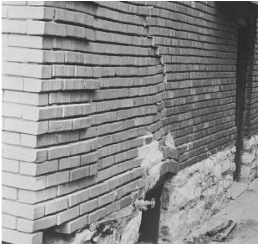
An extreme case of structural failure in a masonry wall due to foundation settlement. The wall and foundation must be completely rebuilt.
