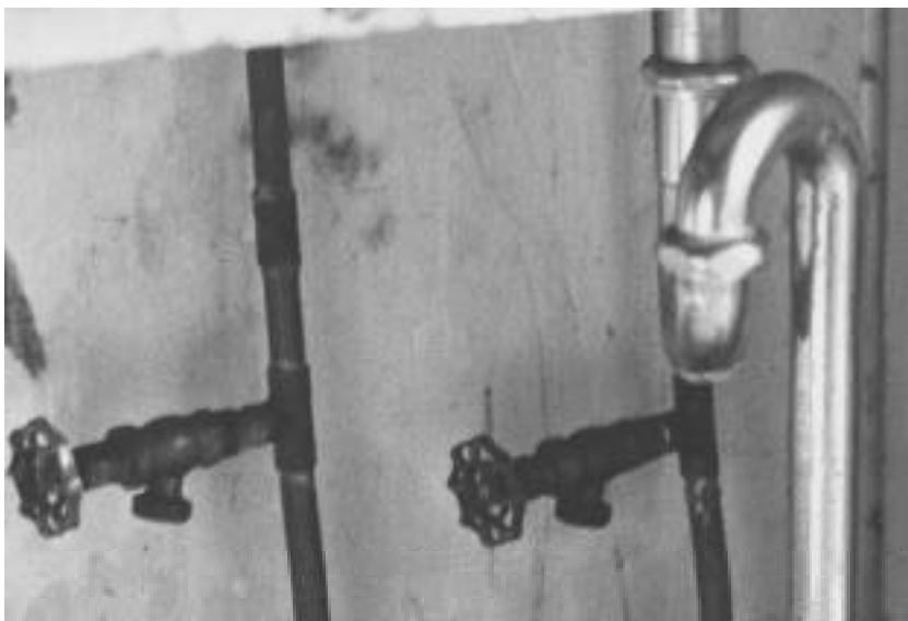
An S-trap that can cause self-siphonage and loss of the water seal. All such traps should be replaced.
