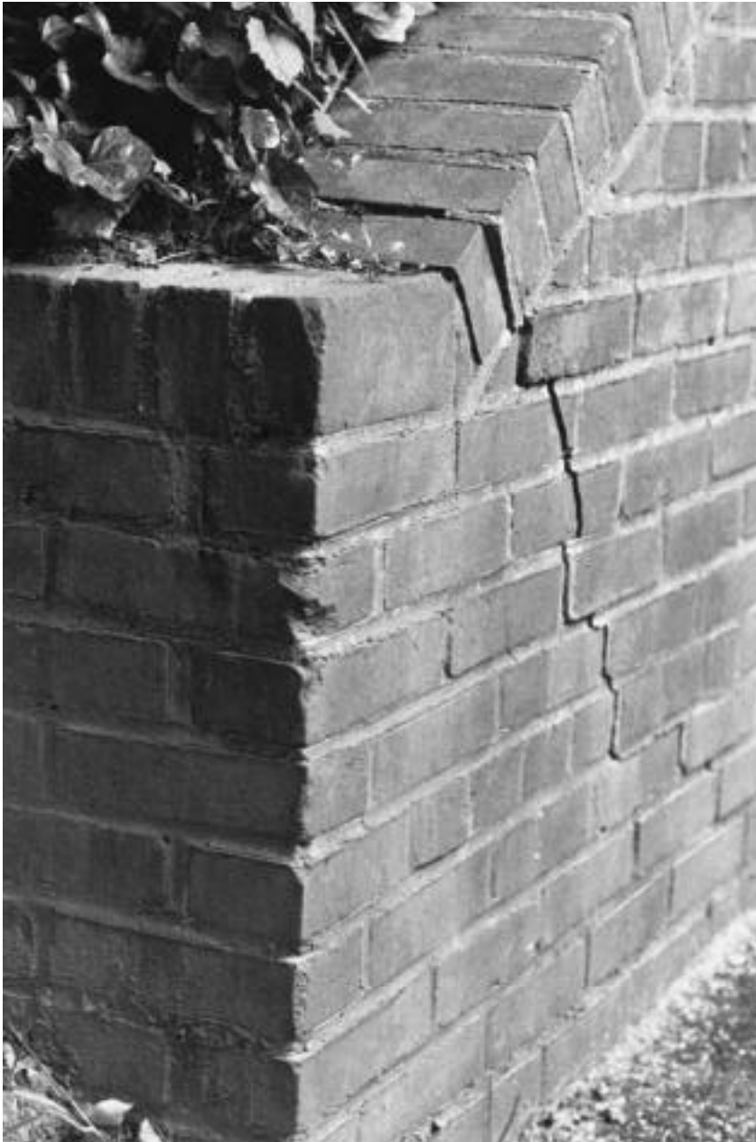
The outward movement of the upper part of this retaining wall can be halted only by structural reinforcement. Simply patching the crack will not solve the problem.
