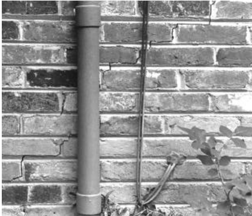
A common masonry wall crack probably caused by thermal or moisture expansion. If possible, monitor such cracks over a period of time to see if they're active. Active cracks should be sealed with a flexible sealant; inactive cracks may be pointed.
