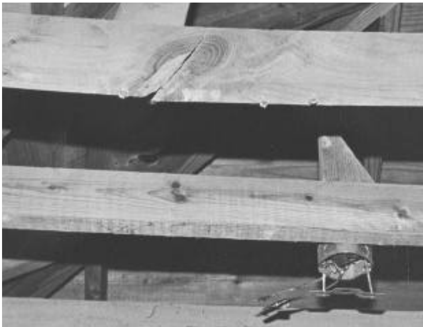
A split ceiling joist or trust chord can be easily repaired by propping it back in place and attaching new structural pieces to each side.
