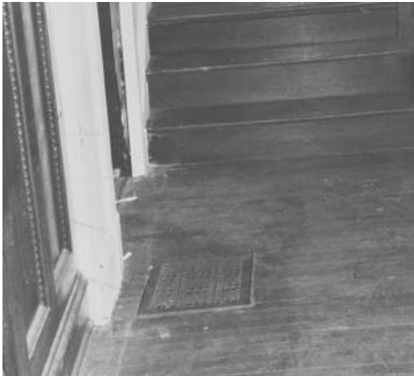
The sagging floor is caused by settlement of a basement support. It may be possible to jack the floor and its adjacent wall into a level position, but this should be done slowly and carefully.
