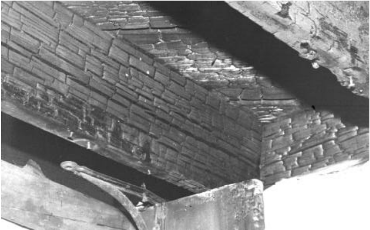
This fire-damaged wood should be carefully probed to determine the extent of charring. In this case, the wood was replaced.
