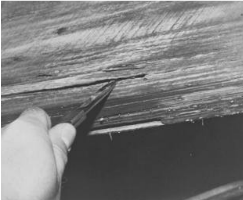
Termite infestation is most common in basements and crawl spaces, particularly near foundation walls. Probe all suspect areas thoroughly.
