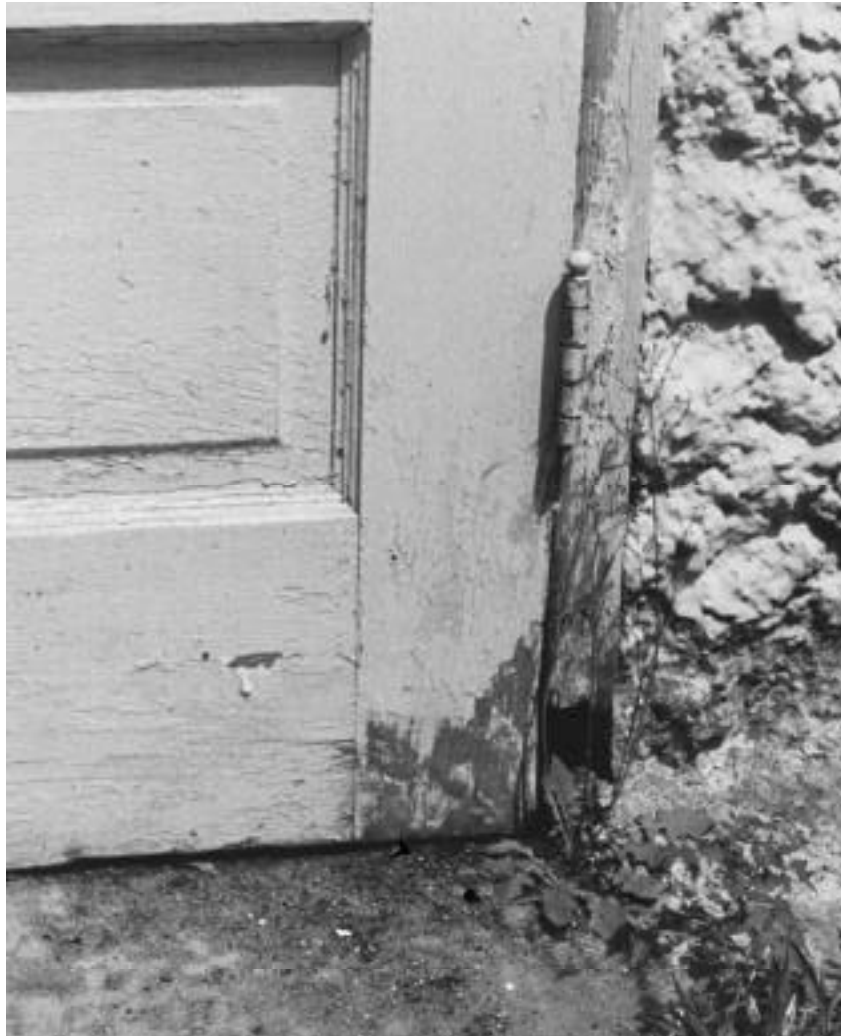
A common location of fungal and insect infestation is where wood door frames touch concrete or earth at grade.
