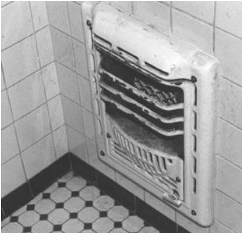
Check the heating source in every room. This particular heater, when tested, was operable and safe.
