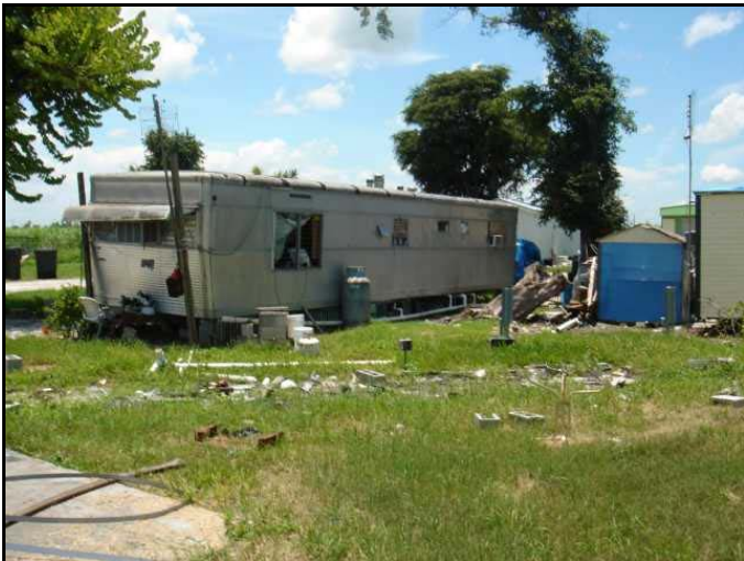
Figure 3 shows an substandard farm worker rental residence in the Glades Communities. This particular mobile home did not have any windows and the yard was covered in debris. Source: CSA, 2006.
