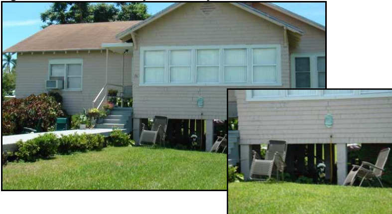
Figure 2 shows a house in the Glades Communities, with an exposed foundation due to the impacts of land subsidence. The second overlay picture shows a close up of the foundation of the house. Source: CSA, 2006.
