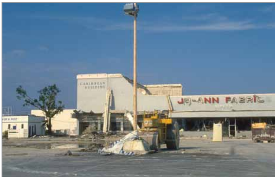
Photo (left): A damaged shopping plaza after Hurricane Andrew. FEMA Photo/ Bob Epstein (August 24, 1992, Dade County, Florida).
