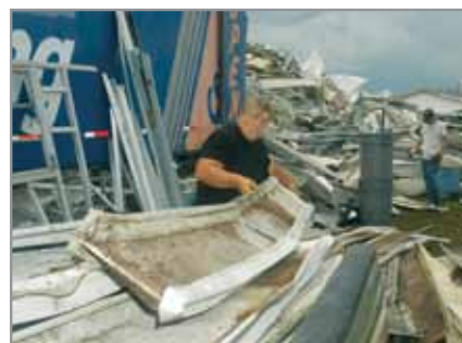
Photo (above): Workers gather aluminum from structures damaged and destroyed by Hurricane Charley for recycling. A debris removal plan that incorporates strategies for recycling and reusing material not only reduces volume at landfills, but also provides more access to materials for rebuilding the community. When developing recycling and reuse strategies, communities should not only include processes for separating these types of materials out, but also a process for making them available to the community. FEMA Photo/Mark Wolfe (August 27, 2004, Hardee County, Florida).
