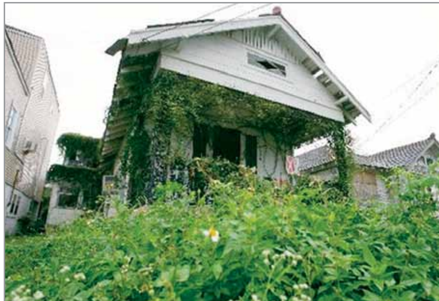
Photo (above): Since Hurricane Katrina, blighted houses have become dangerous eyesores in neighborhoods throughout New Orleans, some threatening collapse. Source: The Times-Picayune.
