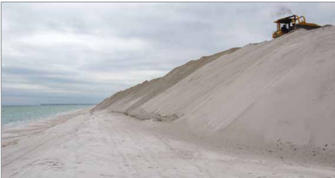
Photo (left): A bulldozer works to repair the sand dune on Pensacola Beach. The dune was destroyed by Hurricane Ivan. FEMA Photo/Mark Wolfe (December 4, 2004, Pensacola Beach, Florida).
