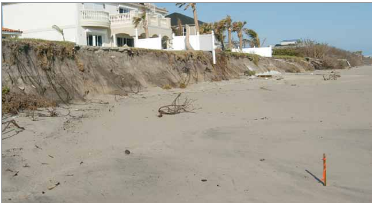
Photo (left): A stake shows the previous extent of the property that was eroded away by the storm surge and wave action of Hurricane Jeanne. (Floridana Beach, FL, October 26, 2004 FEMA Photo/Mark Wolfe).
