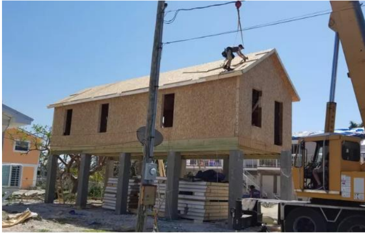
Rebuilding affordable housing on Big Pine Key (Source: A. Cobb, Florida Keys Community Land Trust)
